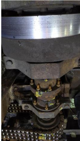
Picture 1: Location of the broken bearing
