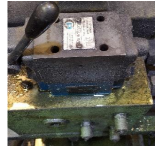
Huge leakage found at the base after cleaning.
